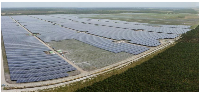
Figure 6. The 300 MW plant in construction in Cestas, near Bordeaux. The modules have a East-West orientation to exploit the sun radiation from early morning to late evening [Reproduced from Ref 28, with kind permission].
