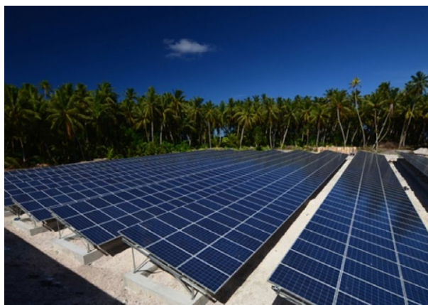
Figure 5. The PV plant in the Atafu atoll of Tokelau island chain in the Pacific Ocean. The world's first territory to become energy-independent with solar PV coupled to storage via lithium ion batteries [Reproduced from Ref 21, with kind permission].
