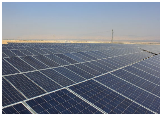
Figure 3. The Dead Sea Photovoltaic Generating Plant, near Jericho, since late 2014 produces electricity dispatched to Jerusalem. Low-cost solar electricity has significantly reduced the cost of the kWh paid by households [Reproduced from Ref 14, with kind permission].
