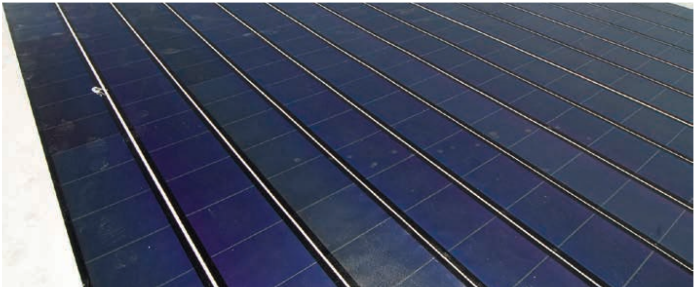
Fig 2 Thin film PV mounted on roof
